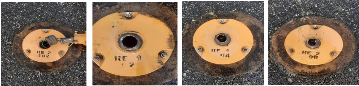
Figure 8 – Damaged runway edge lights
